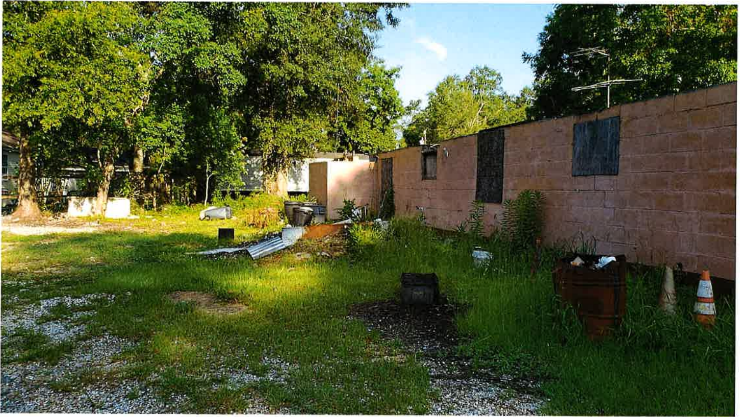
Building to be repaired/demolished
