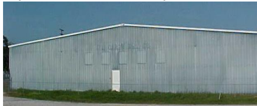
(Example of an unacceptable metal building)
