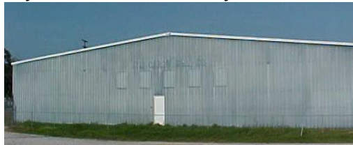
(Example of an unacceptable metal building)
